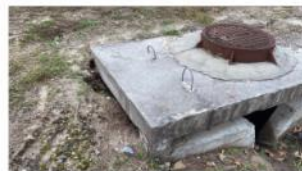
19 OUTLET STRUCTURE EROSION
