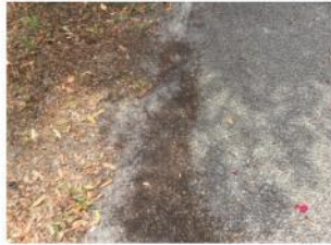
5 UNSTABLE DRAINAGE AREA & 14 DEBRIS (MARGINAL)
