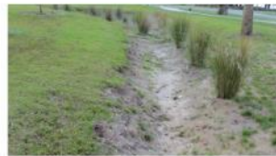
8 INLET EROSION (GRASS CHANNEL)
