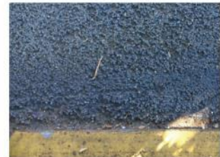
16 SMEARING (POOR) (COVERED WITH ASPHALT SEALER)
