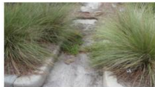
5 INLET STRUCTURE DEBRIS & SEDIMENT
