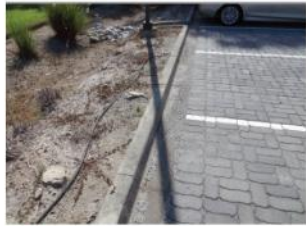
5 UNSTABLE DRAINAGE AREA
