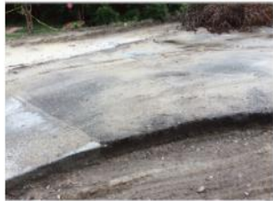
5 UNSTABLE DRAINAGE AREA & 13 SEDIMENT (POOR)
