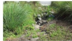
8 INLET EROSION (ROCK PLUNGE POOL)
