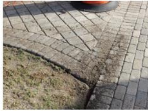
5 UNSTABLE DRAINAGE AREA
