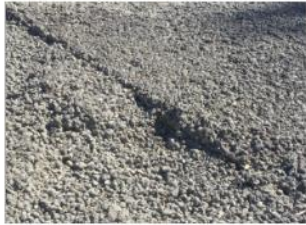
7 CRACKING & 15 RAVELING (POOR)
