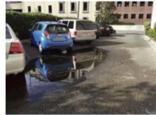
6 PONDING / STANDING WATER
