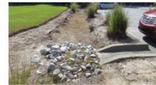
8 PRETREATMENT EROSION (FILTER STRIPS), 14 MULCH (NONE), & 24 PLANT DENSITY (POOR)
