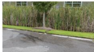
11 EXCESSIVE PONDING (CATTAILS & STAINING)
