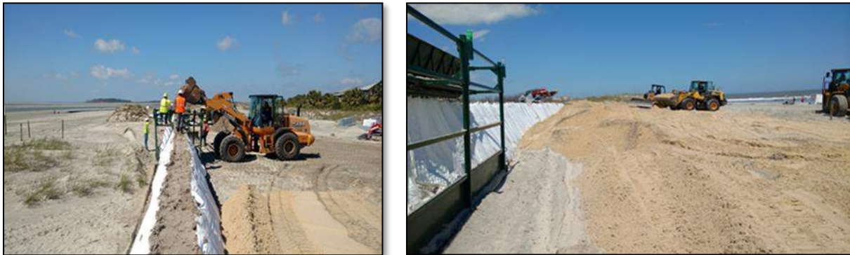
Figure 2.3: PermaShield™ being installed at 19th St on Tybee Island. Photo Credit: Guardian Retention Systems
