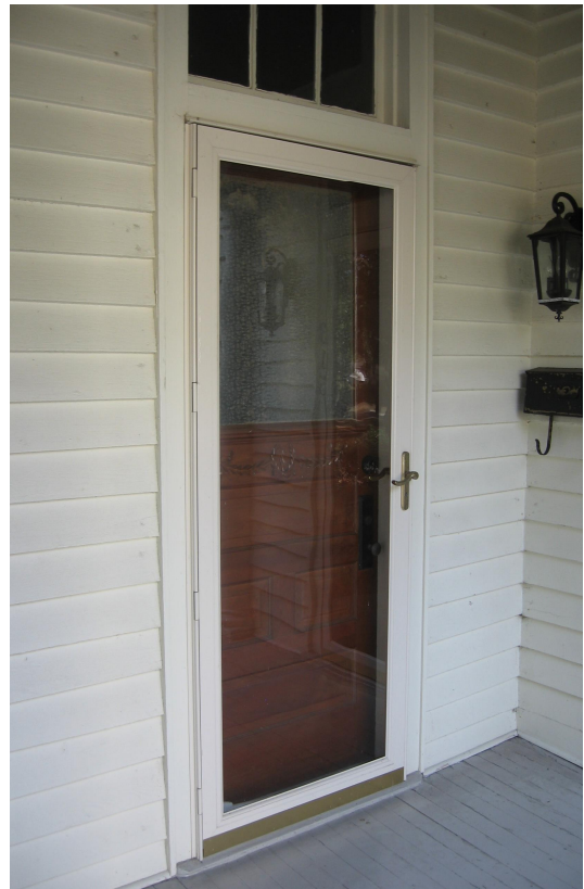
Storm doors should be painted to blend in with the house color and allow viewing of the historic door behind it.
