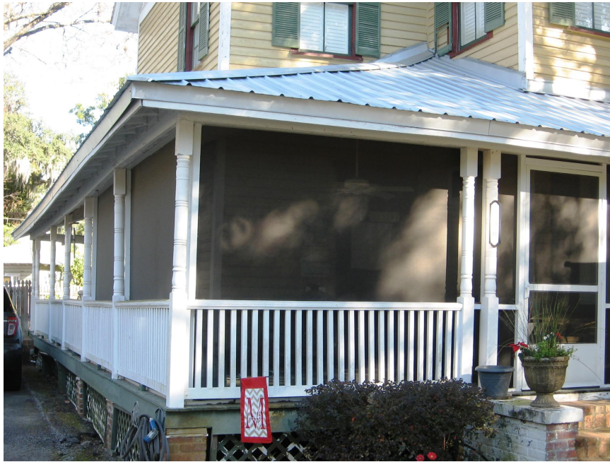
This porch at 706 Union Street is appropriately screened with the panels set behind the porch railing and columns.
