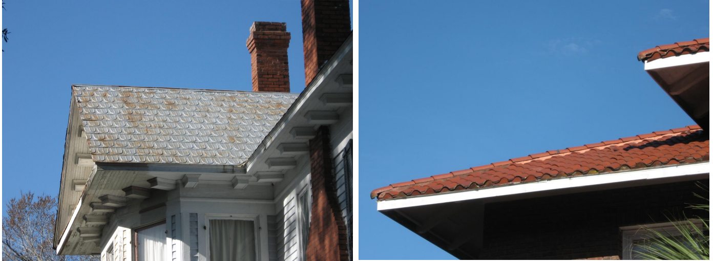
Preserve and maintain original roof surfaces such as the pressed metal shingles at 923 Union Street (left) and the clay tile roof at 826 Union Street (right).
