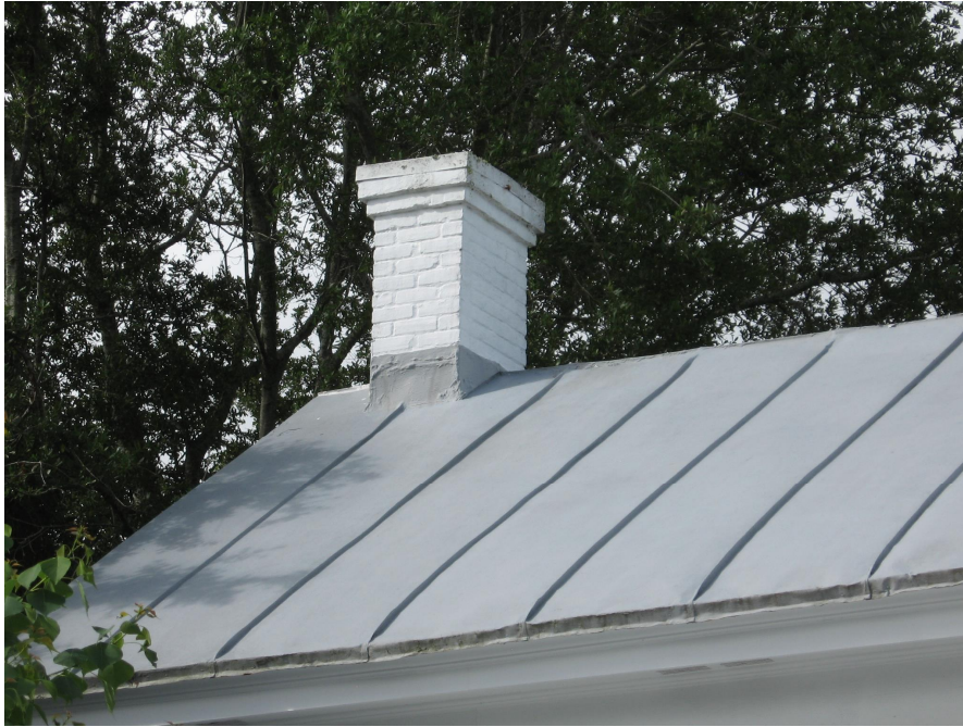
Original standing seam metal roofs are distinguished by their low profile seams.
