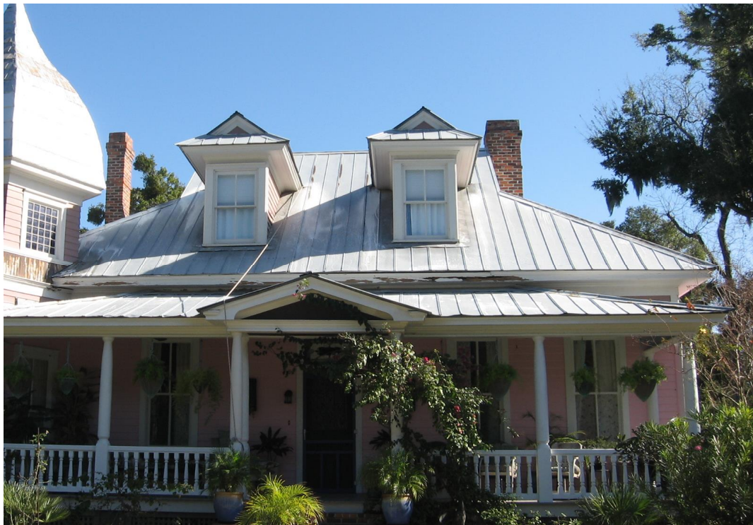
New crimped metal roofs should match the traditional profiles of crimping and spacing as at 1028 Richmond Street.
