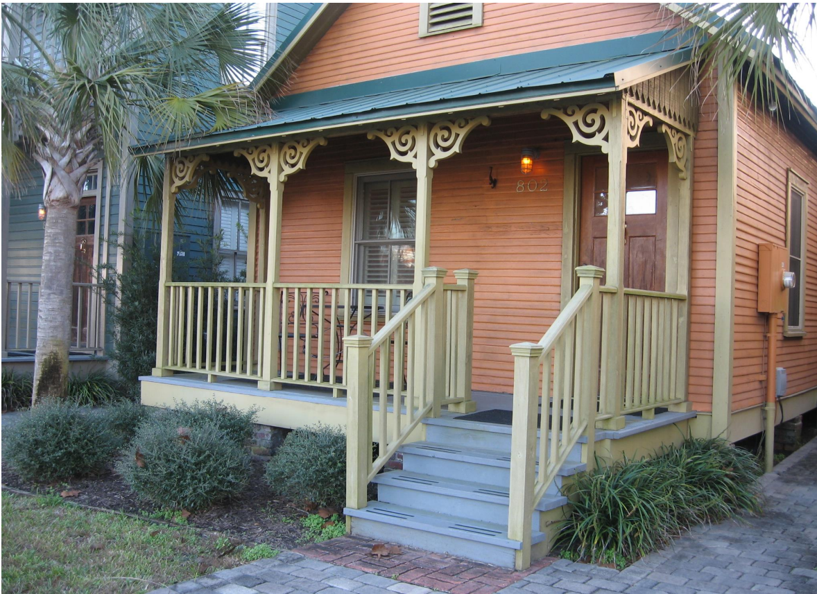
The rebuilt porch at 802 Howe Street displays appropriate wooden steps, hand rails, and balusters.
