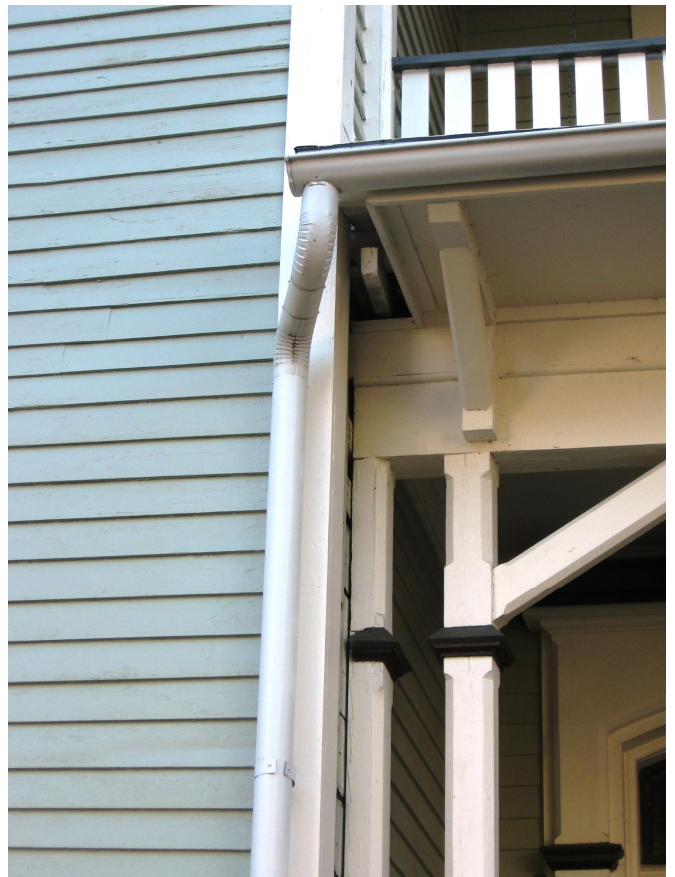
Examples of appropriate gutter and downspout design and locations include 900 Carpenter Street (above) and 927 Union Street (right).
