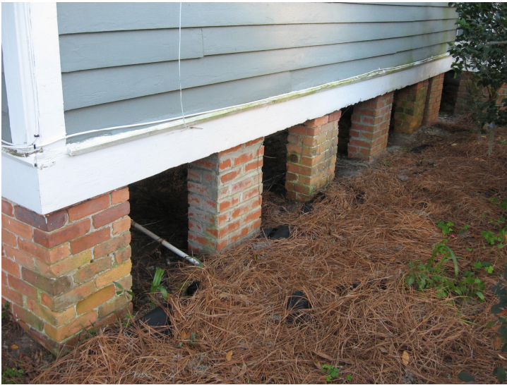
Brick pier foundations should be repointed as needed and left exposed and not concealed (1028 Union Street).
