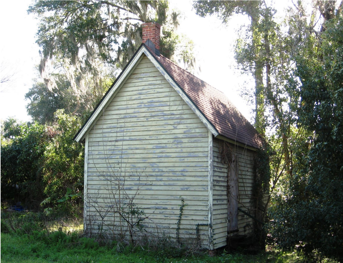
Preserve and maintain original 19th century outbuildings such as this servant's quarters at 502 London Street.
