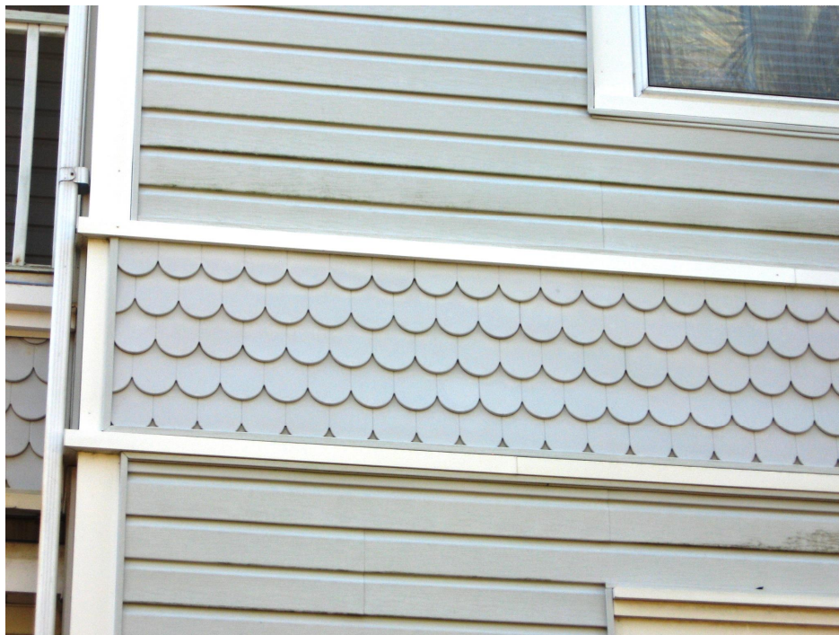
Many dwellings have contrasting siding and decorative wood shingles as at 527 Union Street.
