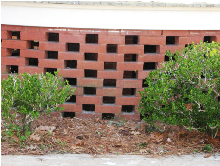
Original pierced brick panels between piers should be preserved and maintained (721 Union Street).
