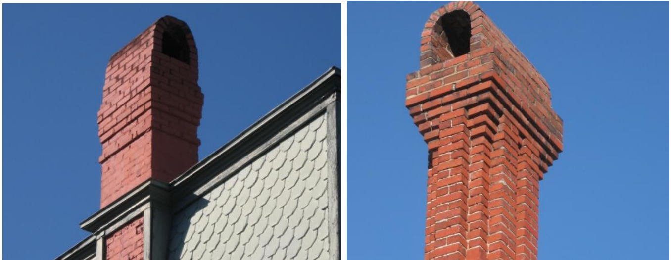
Corbelled brick chimneys can be important features which help define a dwelling's architectural style such as the chimneys at 811 Union Street (left) and 924 Union Street (right).
