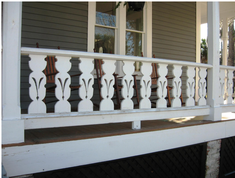
Preserve and maintain detailed porch woodwork as at the dwelling at 928 Union Street.
