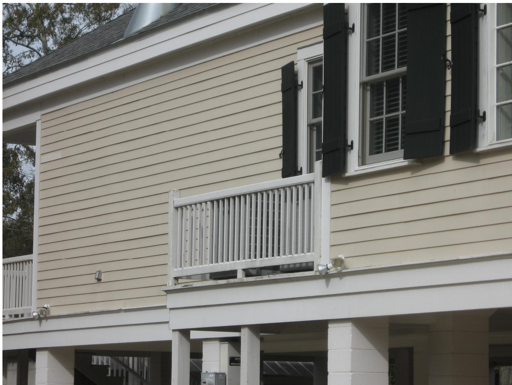
Elevated HVAC units should be placed on platforms or at rear elevations.
