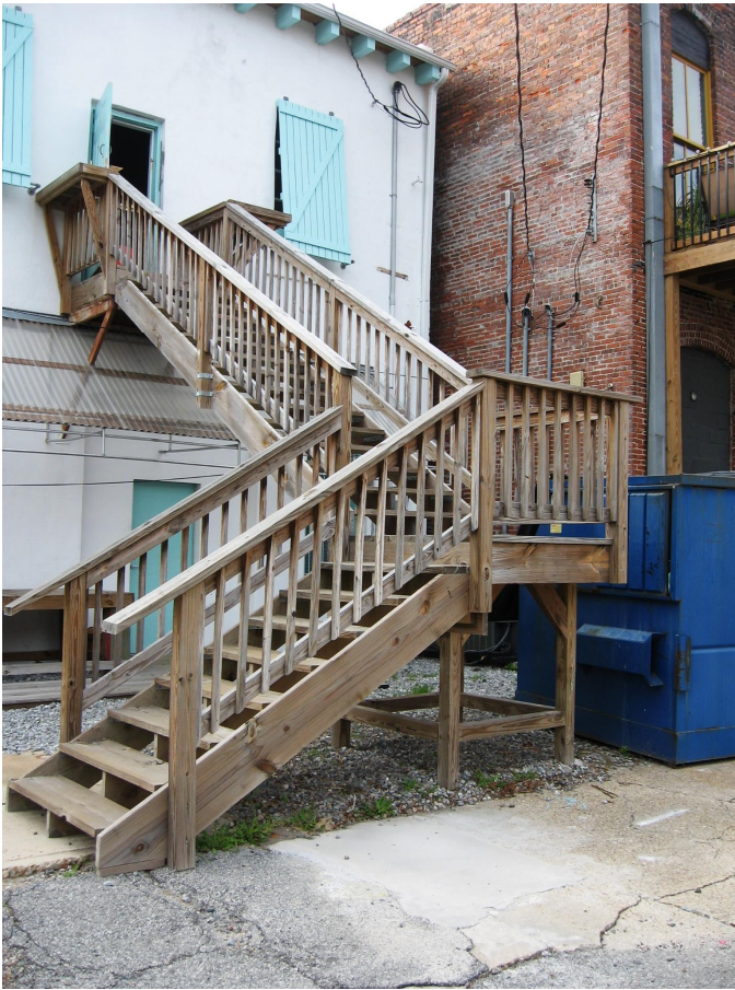
The building at 1602 Newcastle Street has an appropriately designed fire stair of wood construction with square balusters.
