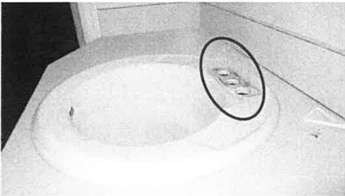
Back bath sink faucet missing
