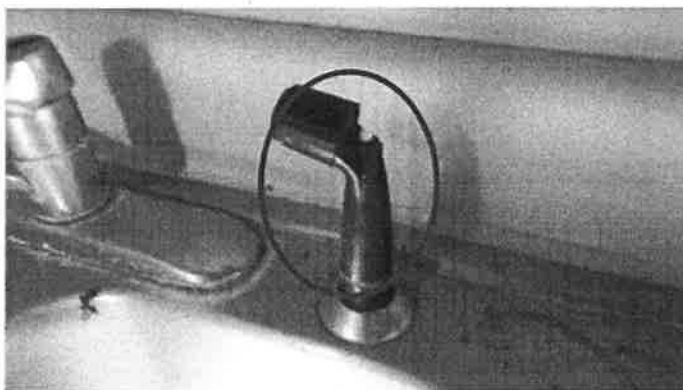
Kitchen sink faucet sprayer damaged
