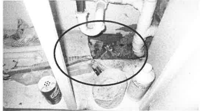
Vanity in bunkroom bath deteriorated, damaged inside
