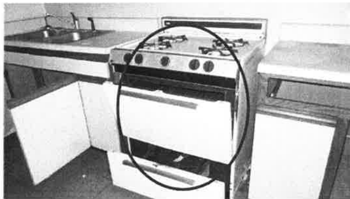
Range, not tested – no gas; worn and near end of life
