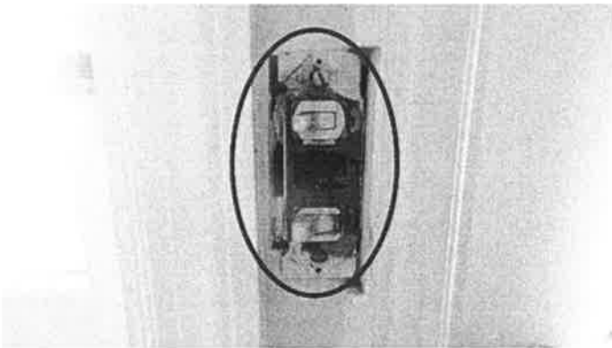
Missing switch cover plate in front lobby area
