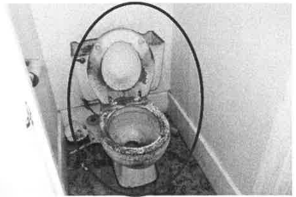
Both toilets at end of life, missing tank covers
