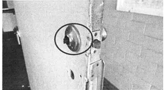
Some interior door knobs broken / missing
