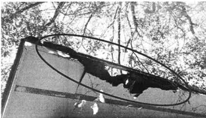
Left side back roof, fascia and soffit heavy damage
