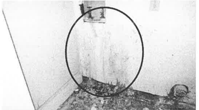
Laundry area wall moisture damaged y water supply pipes
